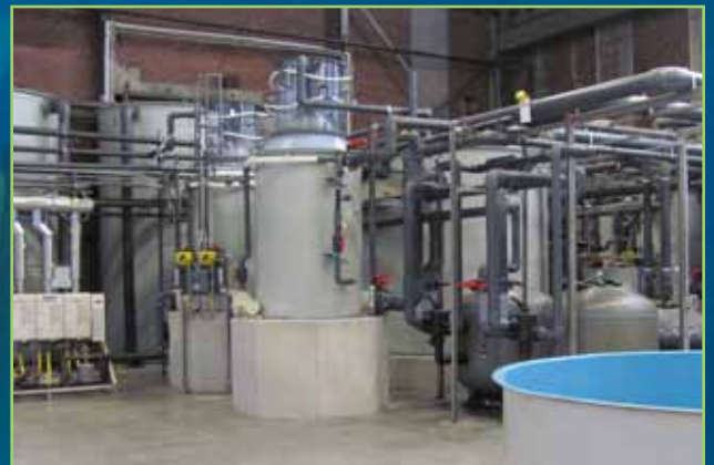
The water-filtration system at the Aquarium's new facility in Quincy.
